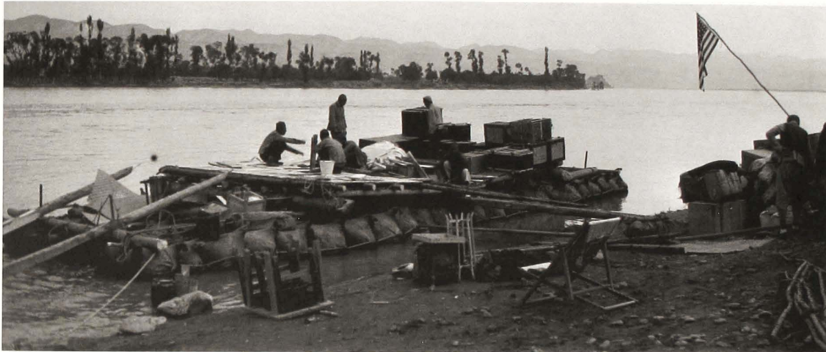
Construction of the raft for the Central China Expedition to return to Paotow, Lanchow, October 1923.
